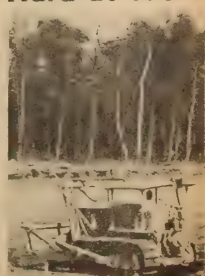
Still hard at work, tractors are digging up land and starting the construction work for more buildings on the new Laval campus. The campus will be open to students in some of the faculties this fall.
